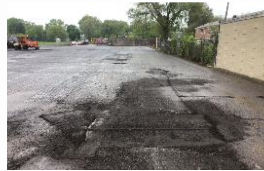
Area Requiring Additional Work
