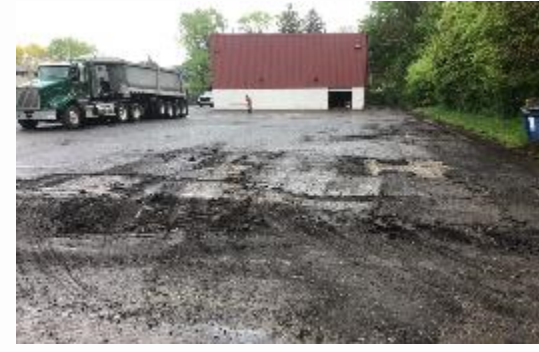
Area Requiring Additional Work
